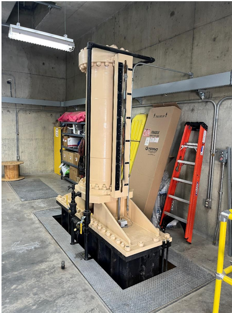
Figure 1. Outlet works jet flow gate and hydraulic piping.
