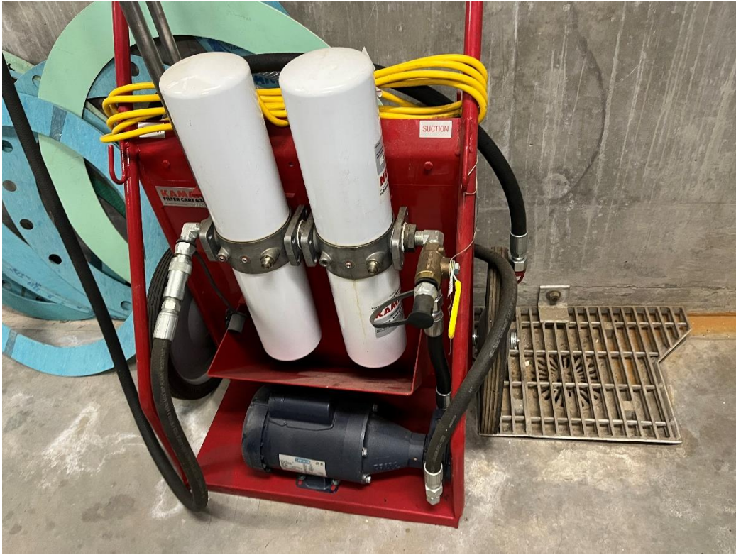
Figure 6. Existing Hydraulic Fluid Filter Cart
