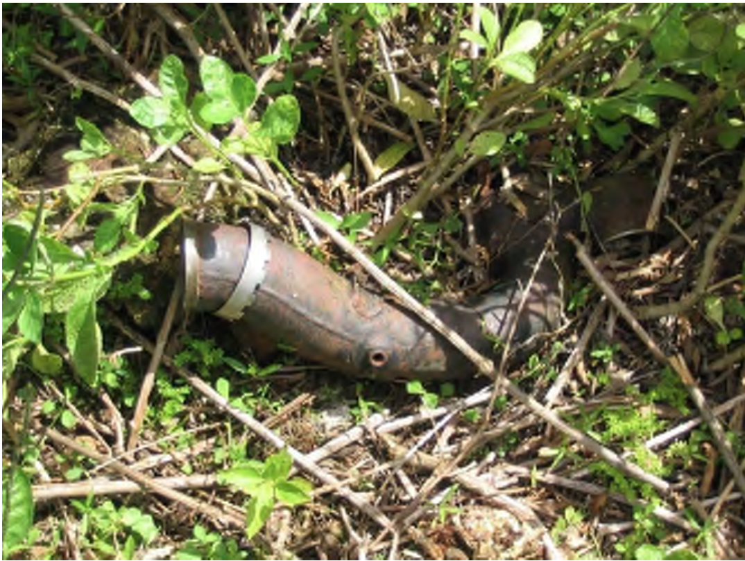
Figure A.3. Pipe located at Site 78, Andersen AFB, Guam
