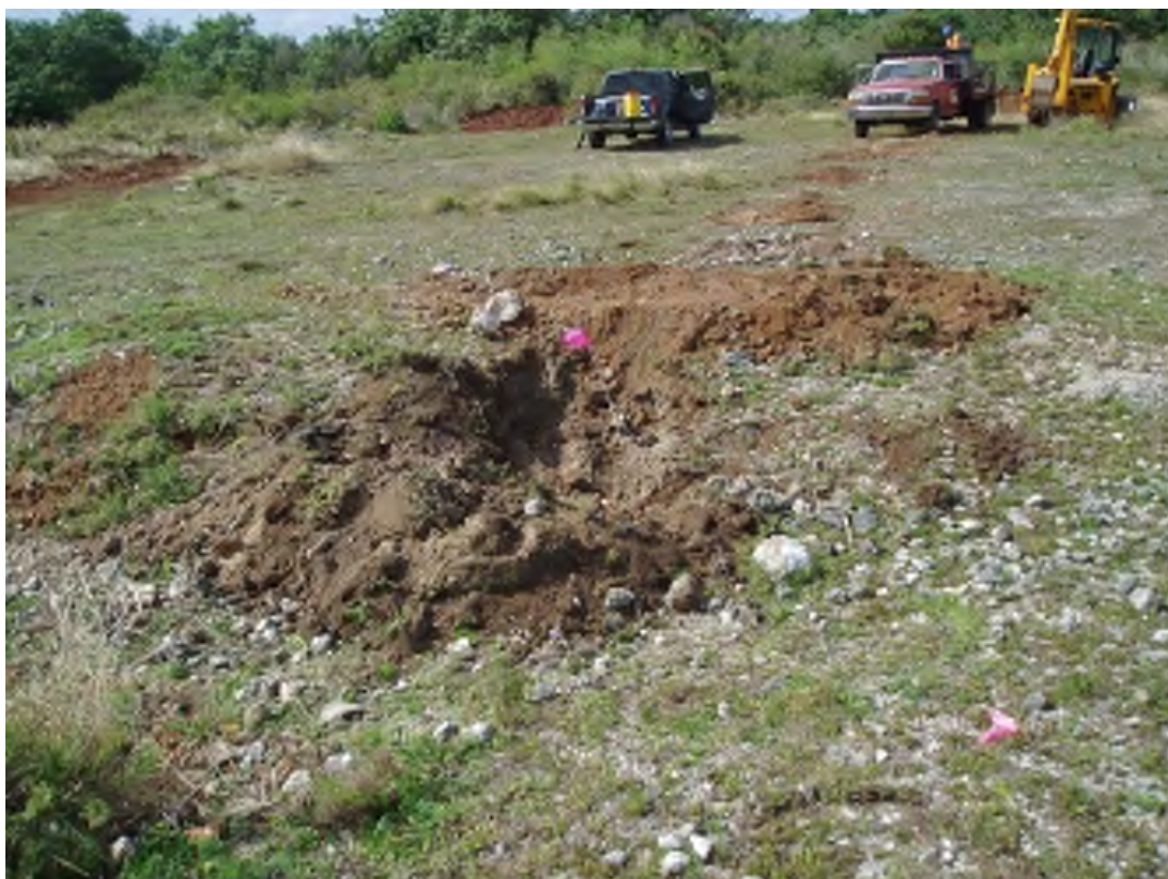
Figure A.11. Pipe leading to the inside of the berm at Site 78, Andersen AFB, Guam
