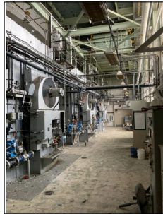
33 G33 - BOILER AREA SCALE: NO SCALE REF DWG: G1004
