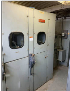
24 G24 - ELECTRICAL ROOM SCALE: NO SCALE REF DWG: G1004
