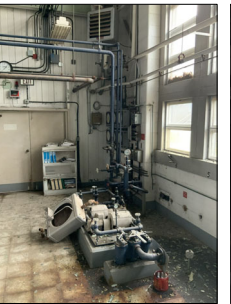
41 G41 - BOILER AREA SCALE: NO SCALE REF DWG: G1004
