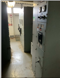
23 G23 - ELECTRICAL ROOM SCALE: NO SCALE REF DWG: G1004
