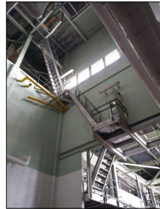
35 G35 - BOILER AREA SCALE: NO SCALE REF DWG: G1004
