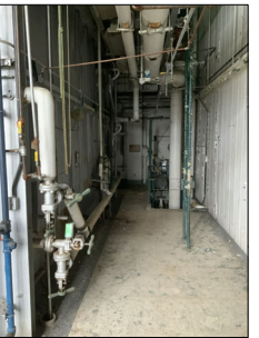
40 G40 - BOILER AREA SCALE: NO SCALE REF DWG: G1004
