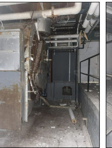
44 G44 - BOILER RM 108 SCALE: NO SCALE REF DWG: G1004
