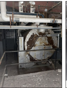
42 G42 - BOILER RM 108 SCALE: NO SCALE REF DWG: G1004
