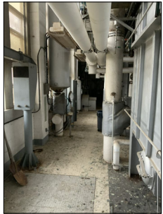
36 G36 - BOILER AREA SCALE: NO SCALE REF DWG: G1004
