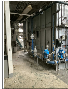
34 G34 - BOILER AREA SCALE: NO SCALE REF DWG: G1004
