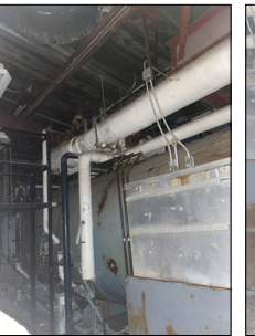
43 G43 - BOILER RM 108 SCALE: NO SCALE REF DWG: G1004
