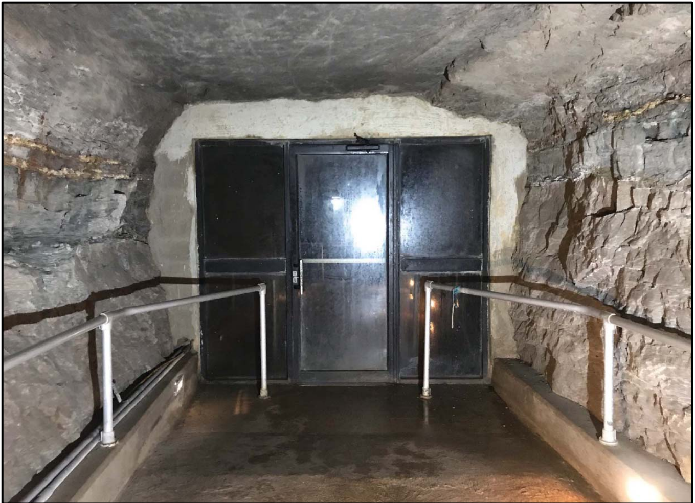
Figure 23: Dripstone Cave Exit – Inner Airlock Door (Existing Conditions)
