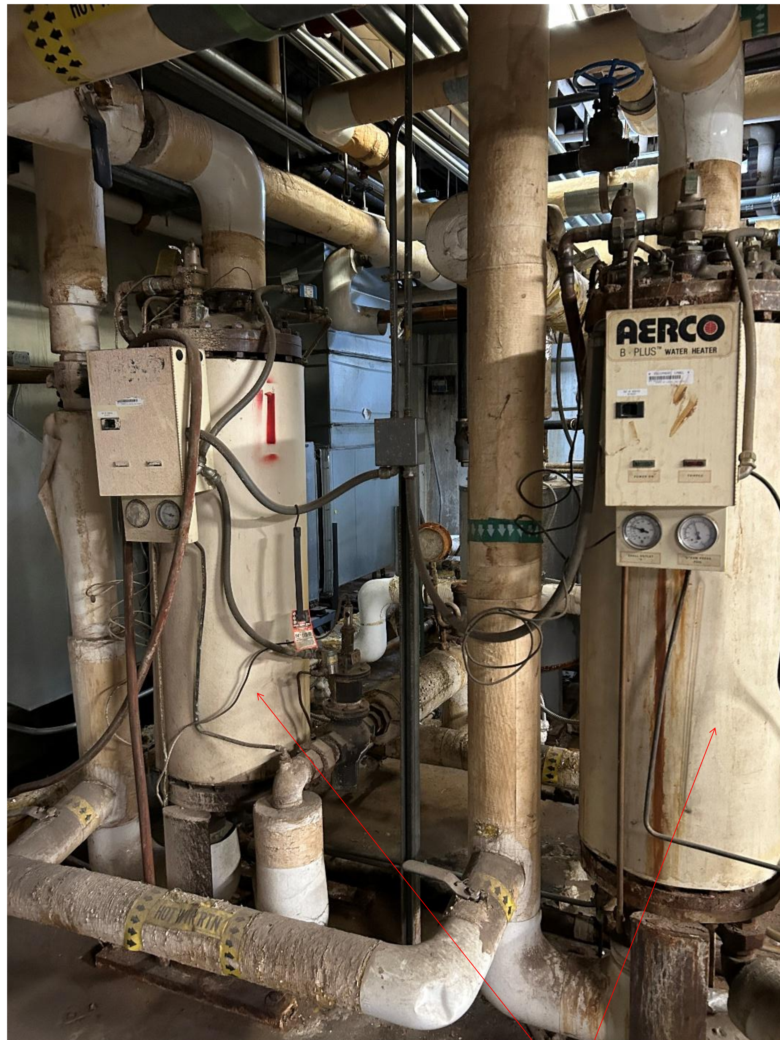
HOT WATER GENERATORS 1 & 2
