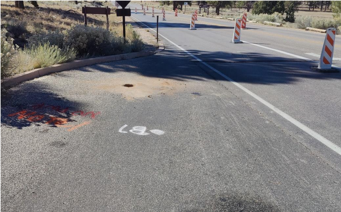
YA-B1 Existing Shuttle Stop – 4 inches of ACP in good condition – Thermal crack and Joint separation at edge of driving lane.
