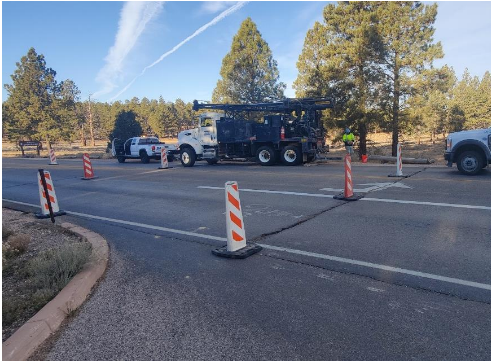
YA-B3 – Only distress large thermal crack and joint crack at edge of driving lane – shoulder boring
