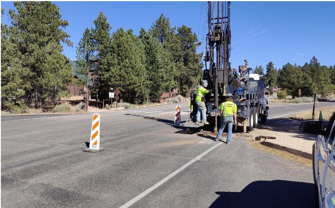
YA-B2 – Mainline Pavement Northbound – 4 ½ inches of ACP – Only one Thermal Transverse Crack – Pavement appears to have recently received a chip seal
