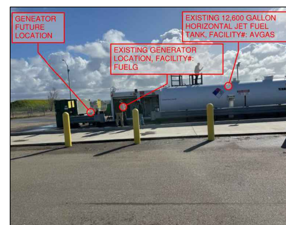
G10 EXISTING AND FUTURE GENERATOR LOCATION (LOOKING EAST) SCALE: NO SCALE
