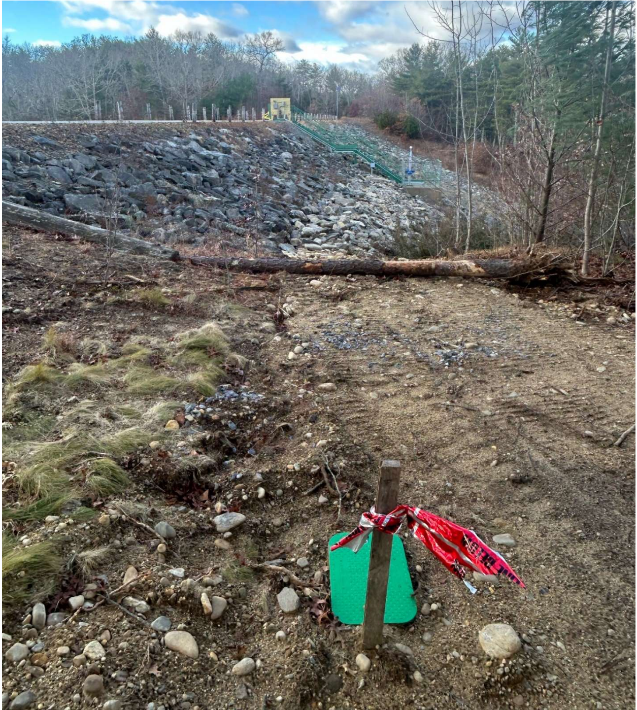
Image 5: Photo showing the generator pull box in line with the pull box on the stairs. 130' of conduit is ran from this point across to the stairs.
