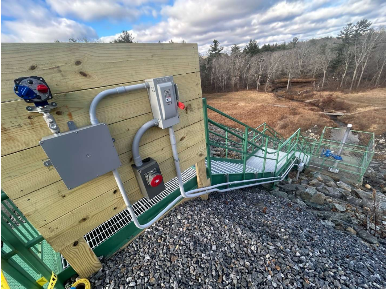
Image 7: Photo showing existing control panel at top of dike. Electrical connections are to be ran from generator to pull box, then up to these controls. Existing generator connection will be removed.
