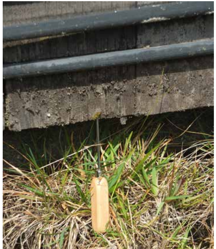
Figure 12: Wood is most vulnerable to water penetration at the end grain, yet even in areas where grass was growing directly under the ends of the staves, an icepick would penetrate less than an eighth of an inch, indicating that the staves remain in good condition.
