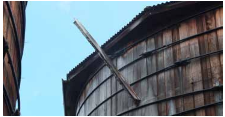
Figure 23: The remaining gutters are in poor condition and some, as seen here, are detached and dangling precariously above the ground.
