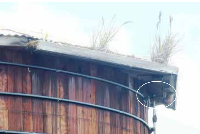
Figure 22: Some tanks retain sections of the original wood gutters. What remains is in poor condition, is choked with debris, and is supporting healthy vegetative growth. Visible here is the gutter's "downspout" (circled). As might be expected, the rain that fell on the tank roofs was also collected and channeled into the tanks.
