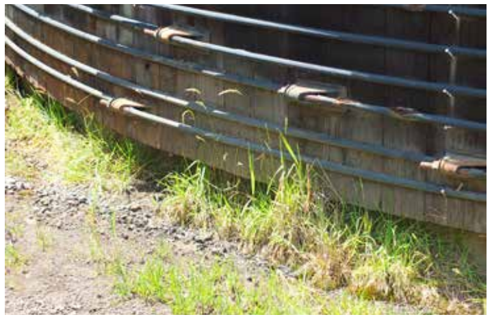
Figure 8: Changes in soil levels have covered the bottom halves of the footings allowing grass to grow right up to the base of the tanks.
