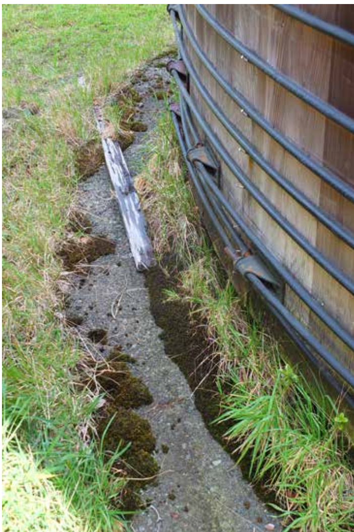
Figure 7: At the base of the tanks, the concrete footing steps back approximately at grade level. Soil deposition has both raised the grade around the tanks and allowed soil to accumulate on top of the footing, supporting the growth of both grass and moss. This will accelerate the deterioration of both the concrete footing and wood staves.
