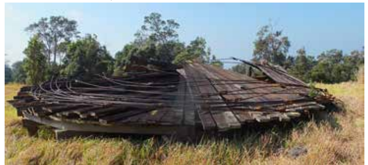
Figure 24: Although a smaller tank in a different location, this clearly illustrates what can happen to an empty tank. With no water in the tank, there is no outward pressure on the staves. As the staves dry and shrink, gaps will open between the staves and, once there is enough space for one stave to fall inward, the rest will quickly follow.
