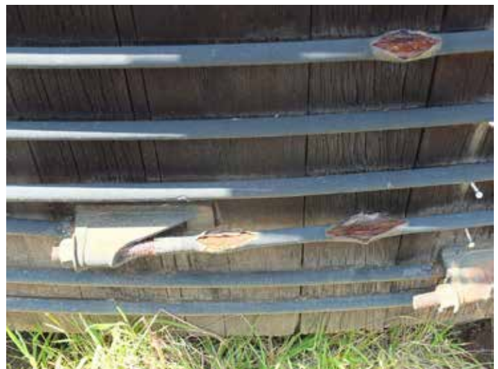
Figure 16: General view of tank bands showing areas of corrosion. Corrosion is widespread with a number of bands having rusted completely through. In addition, all of the threaded ends have corroded to the extent that the bands will need to be cut for them to be removed.
