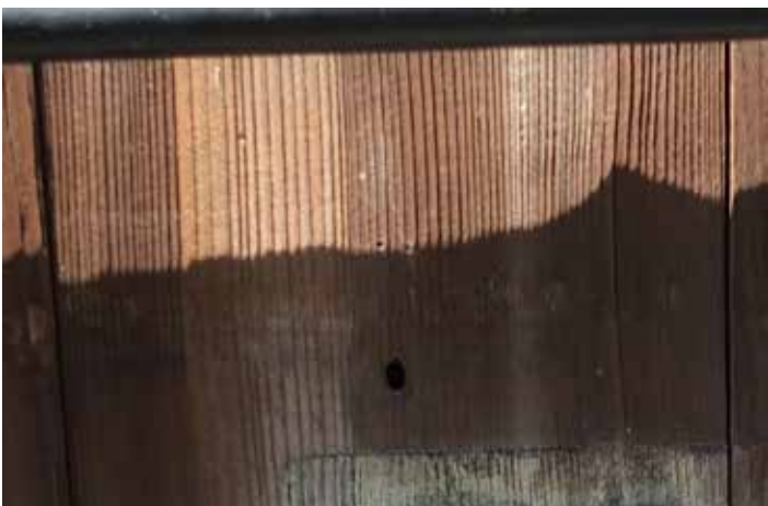
Figure 14: Ultraviolet degradation is one cause of raised grain, as seen here.
