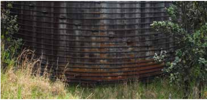
Figure 13: As seen here, close proximity of vegetation, including grass, shrubs, and trees can create microclimates that prevent drying and encourage the growth of moss and fungus on the wood staves. The area around the tanks should be kept clear of vegetation and the grass should be kept short.
