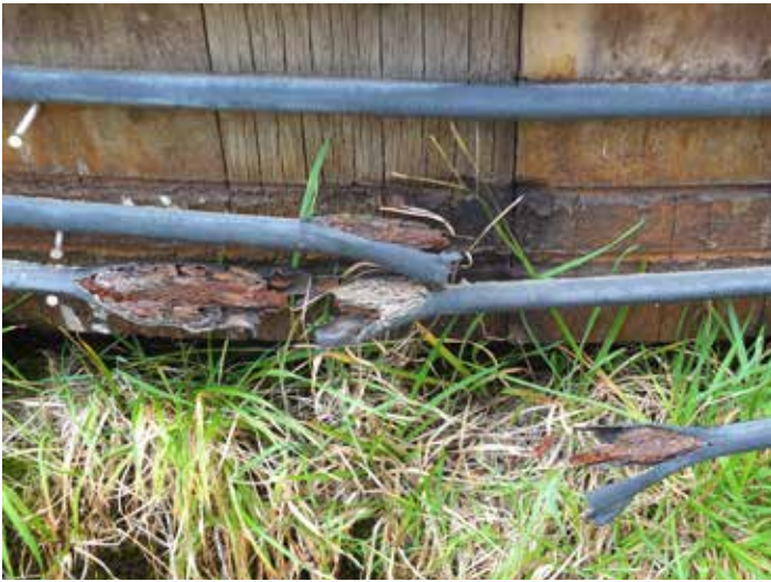
Figure 17: On one tank, both of the bottom two bands have rusted through. Because these two bands compress the staves against the concrete foundation, this tank may be structurally compromised. Compression at the bottom end of these staves should be reestablished as quickly as possible.
