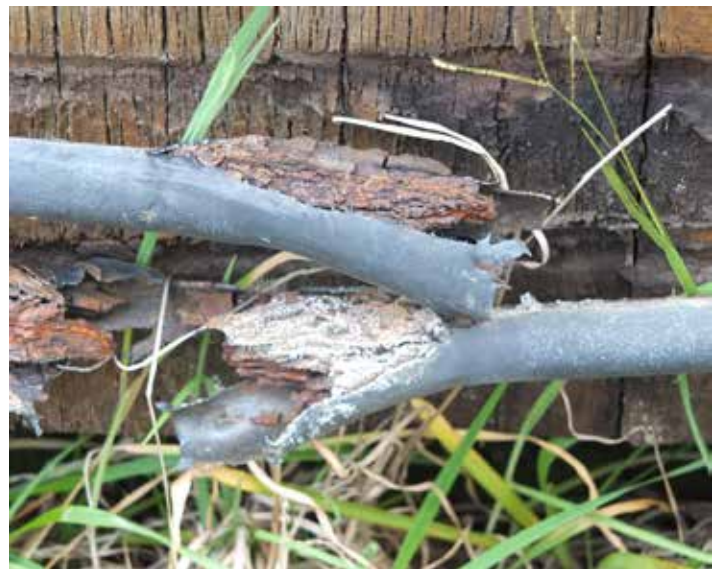
Figure 6: The damp climate, coupled with the presence of sulfur dioxide from volcanic gases, has caused the mild-steel in the tank bands to corrode. Here the band has rusted completely through.
