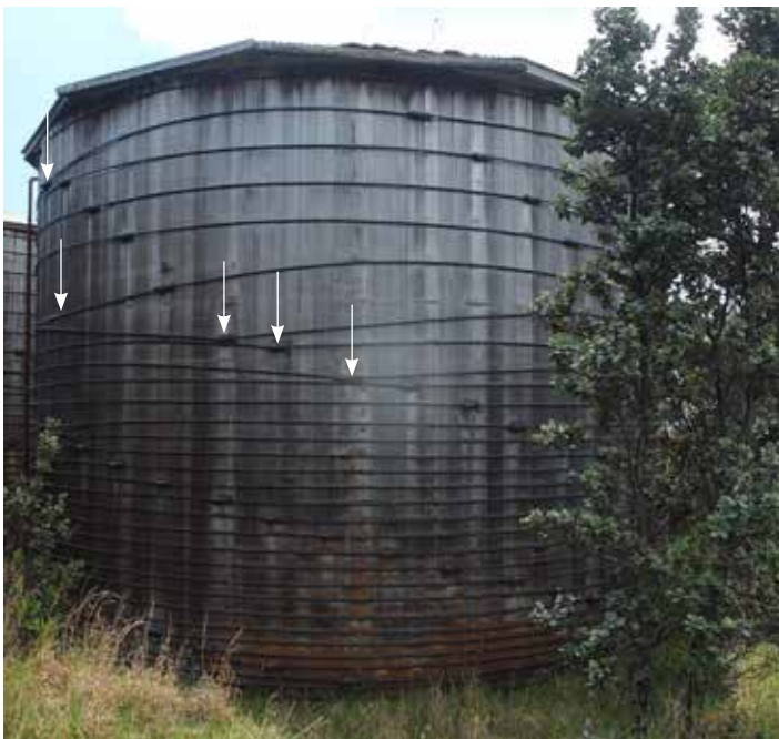
Figure 18: Without the swelling and outward pressure that result from filling a tank with water, the circumference of an empty tank will shrink, releasing pressure on the steel bands. Where the nails supporting the bands have failed, the lugs and bands are slipping downward (arrows).
