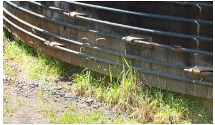
Figure 26: The effects of “splash” are clearly visible here. The line of gravel on the ground that runs along the base of the tank shows where the water from the roof hits the ground. That water splashes back against the bottom of the tank, wetting the bottom ends of the staves. This allows moss and fungus to grow on the wood, leading to deterioration.
