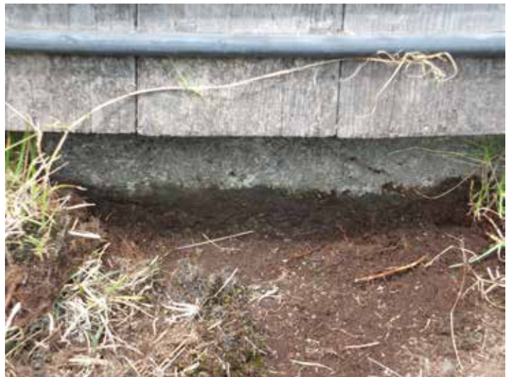
Figure 9: Close-up of the base of a tank showing where soil had covered the foundation's step-back allowing grass to grow on top of the concrete. This condition can potentially accelerate the deterioration of both the wood staves and the concrete.
