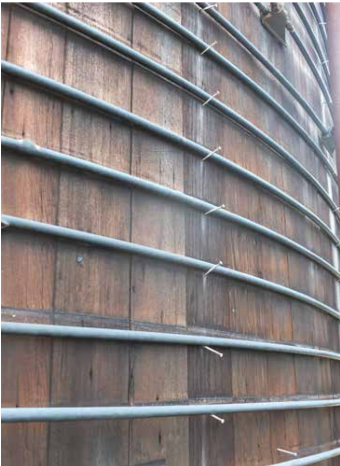
Figure 11: Close-up of tank staves and bands. Note that because the tank is empty there is no horizontal hydrostatic pressure to push outward and hold the steel bands in place. Nails have been used to prevent the bands from slipping down.
