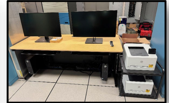
TFDM Monitor & Control (M&C) Workstation, System Support Workstation (SAS-1), OPS and Support Printer
