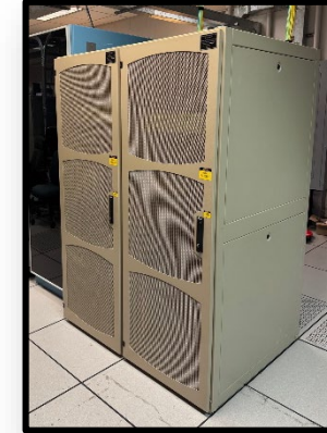
TFDM Equipment Racks
