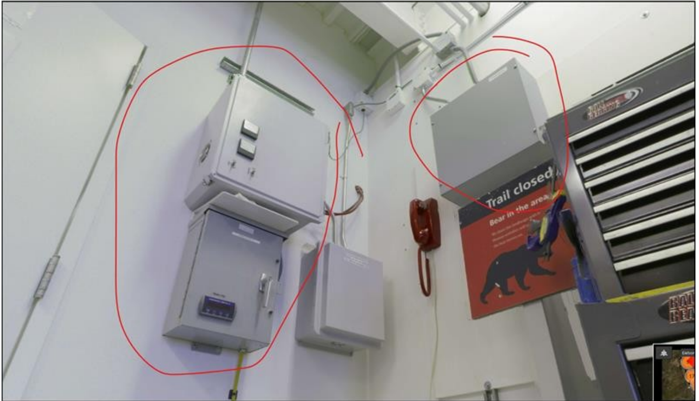
Photo 1 - Utility Building equipment overview. The red circles identify the left-side equipment group and the upper-right enclosure referenced in the following photographs. The red wall phone visible between the equipment groups was reportedly intended for communication with the turbine house; operational status has not been verified.
